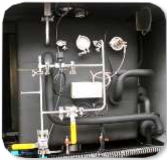
Backside of drying chamber
