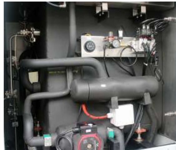
Fluid recycle and electric heater
